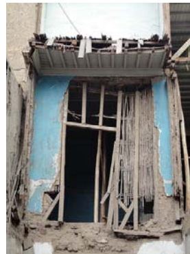
Severe deterioration in upper stories
